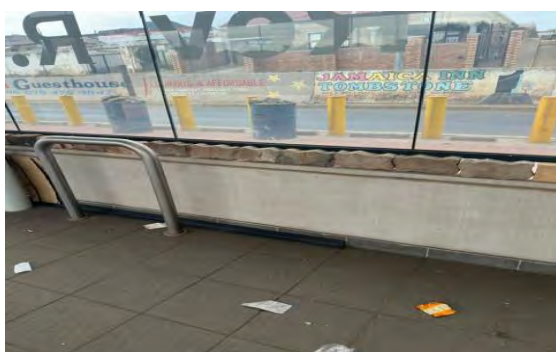
Figure 3: Displaced bricks at MA Mkhwanazi Station and Rev. RTJ Namane station
