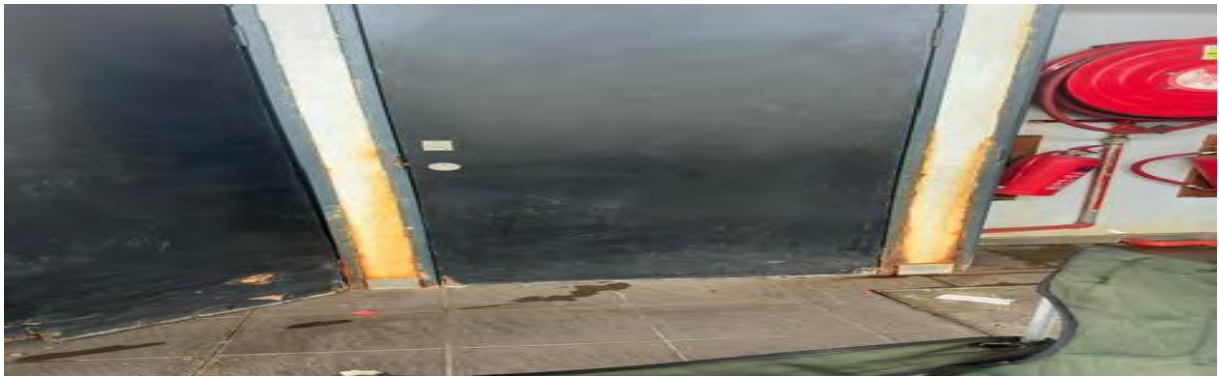
Figure 4: Rusted door frames at MA Mkhwanazi Station
