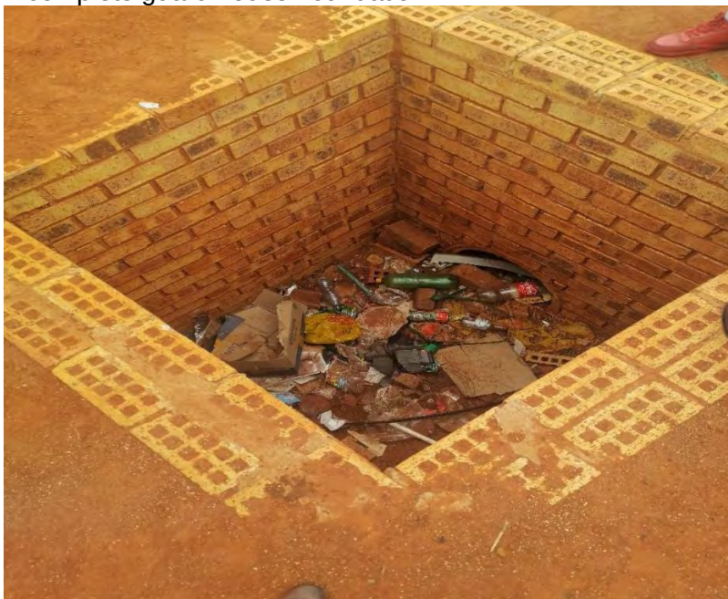
Civil work: open sinkhole
